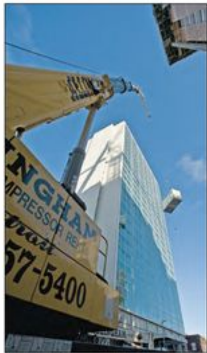
Coupling the jib to the crane's 197-foot-long main hydraulic boom created the long "arm" of latticed steel needed to reach the very top of the Tower Plaza.
